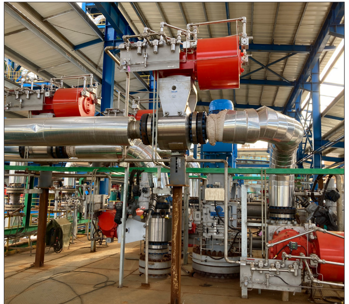
Slurry feed line valves into autoclave consist of NPS 10 (DN 250) titanium isolation valves.
