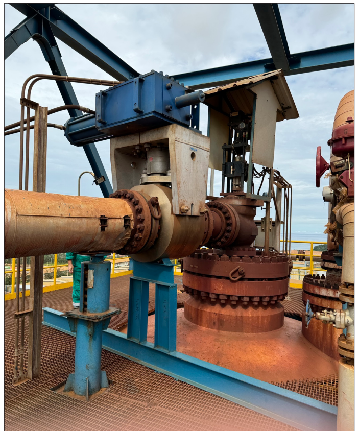
Slurry discharge line of NPS 14 (DN 350) with compact HPU skid into first letdown drum. This is the highest elevation point in the autoclave circuit.
