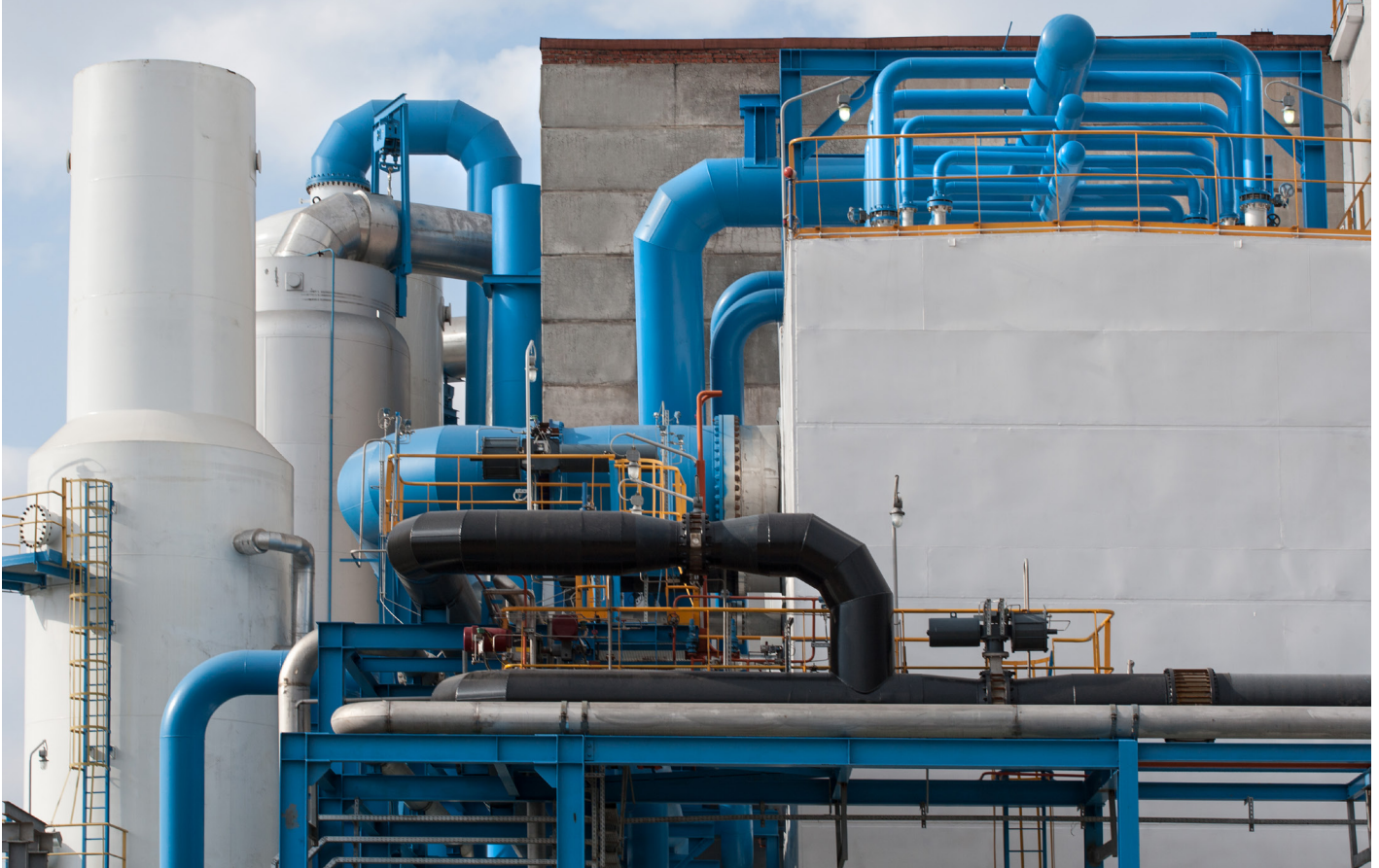
Air separation plant for producing industrial gases.
