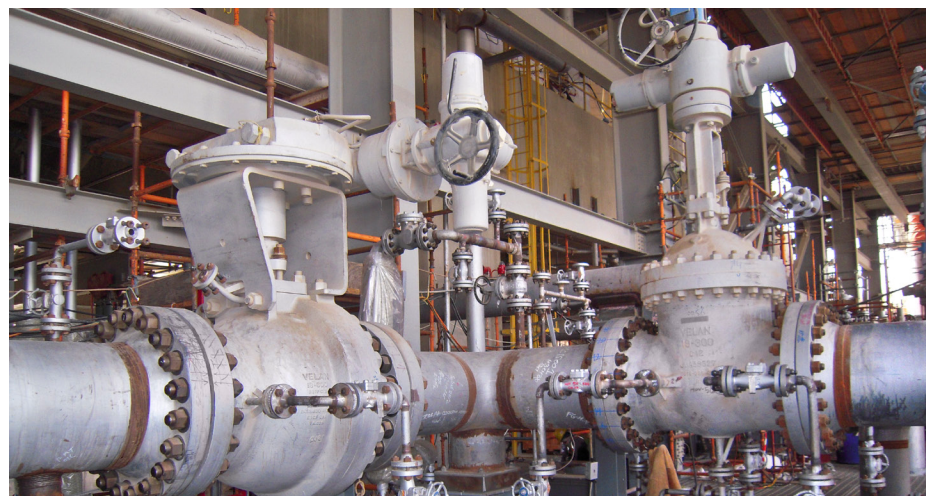
Velan coker valves in pre-commissioning.
